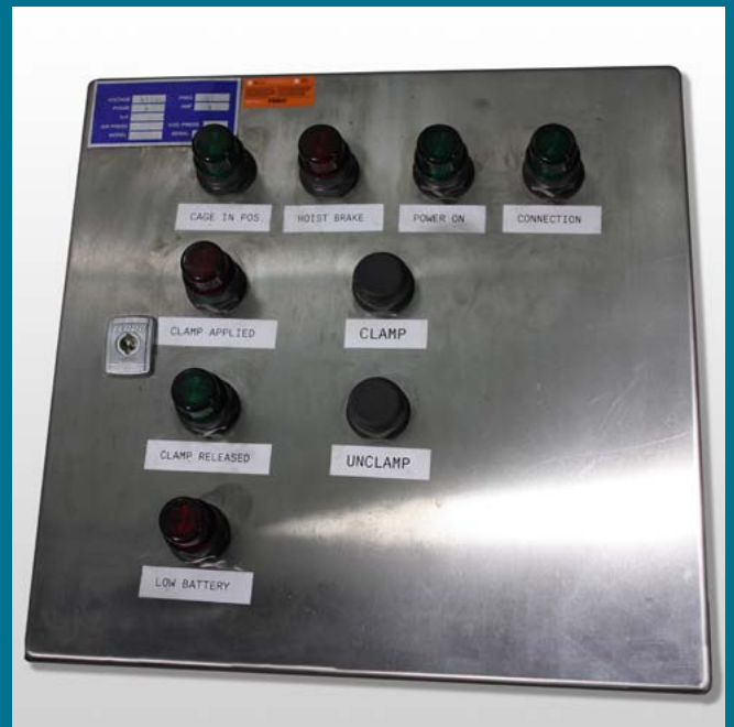
Underground Station Control Panel
